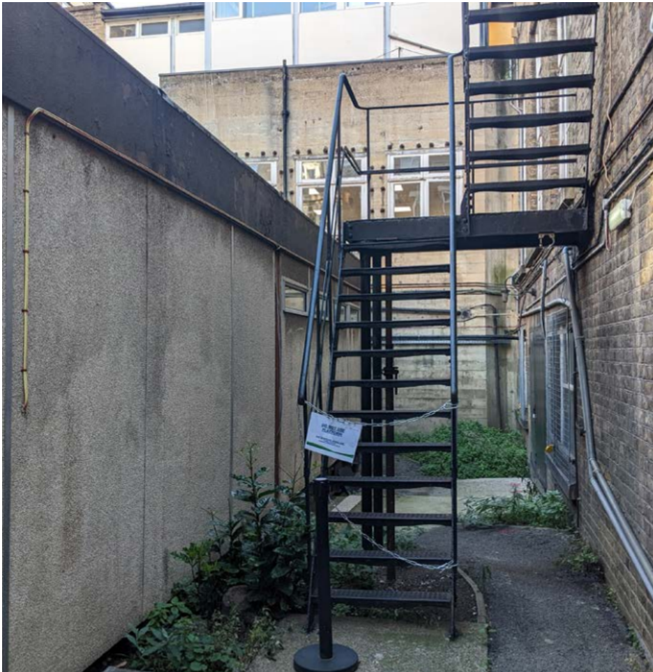
Images 3 & 4: Stair from neighbouring property and out of use sign
